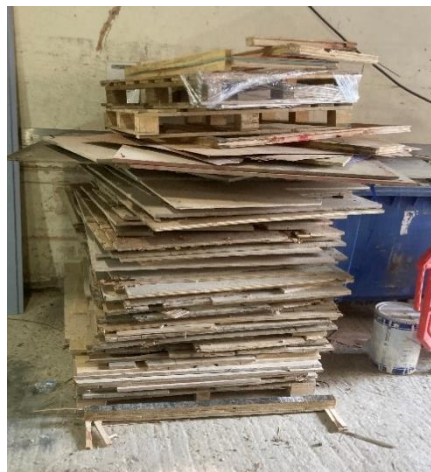
A photo of the plywood that was recovered from the refurbishment project
